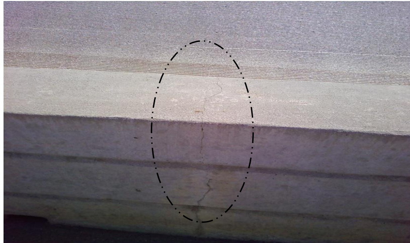
Figure 4.5. Guardrail Transverse Cracking
