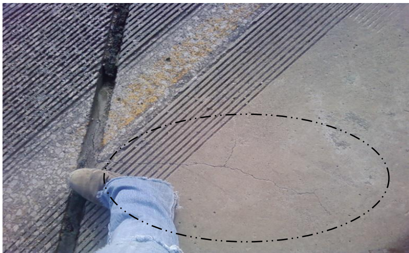
Figure 4.3. Off-Ramp Slab Cracking
