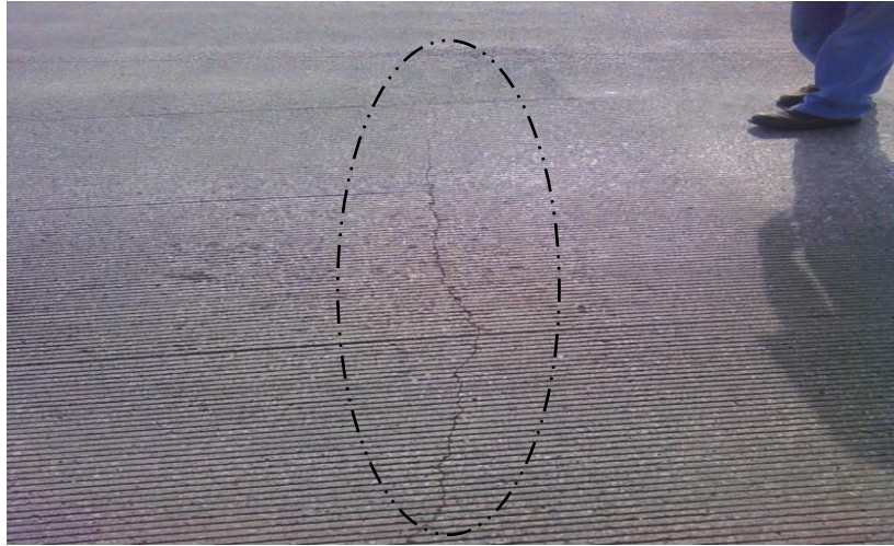
Figure 4.4. Deck Transvers Cracking
