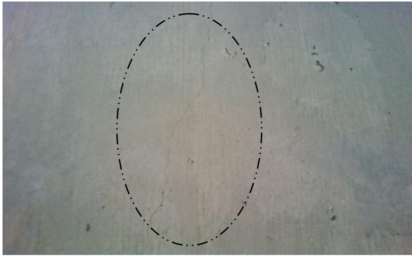
Figure 4.1. North Abutment Hairline Crack
